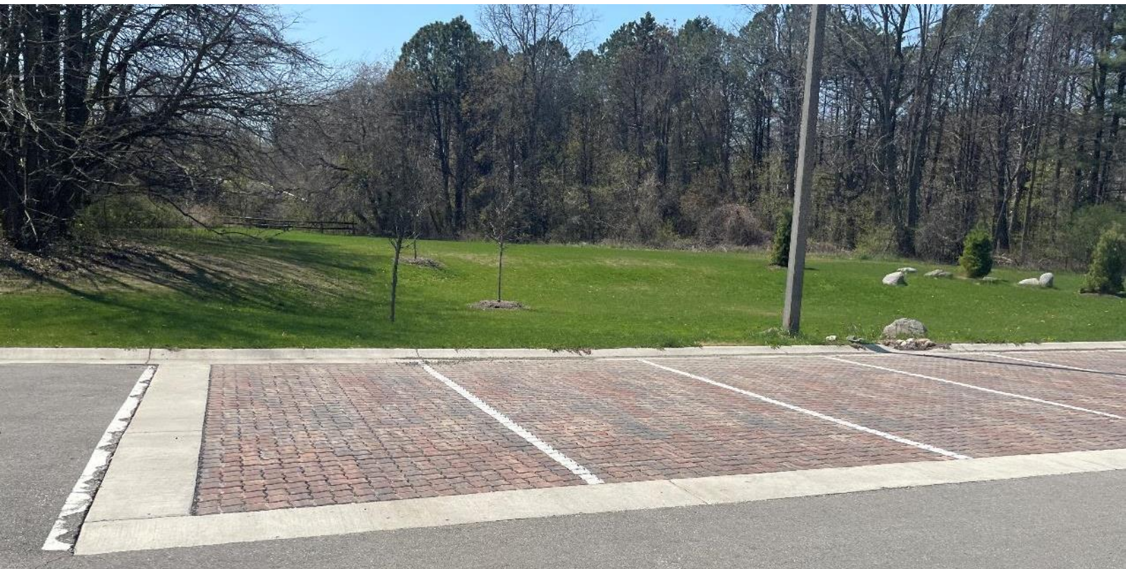
FIGURE 14: Grant Park has already seen the need for stormwater improvements.
