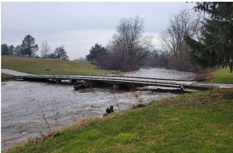
FIGURE 11: Menomonee River Parkway after heavy rains. Image: Andre Ost.
