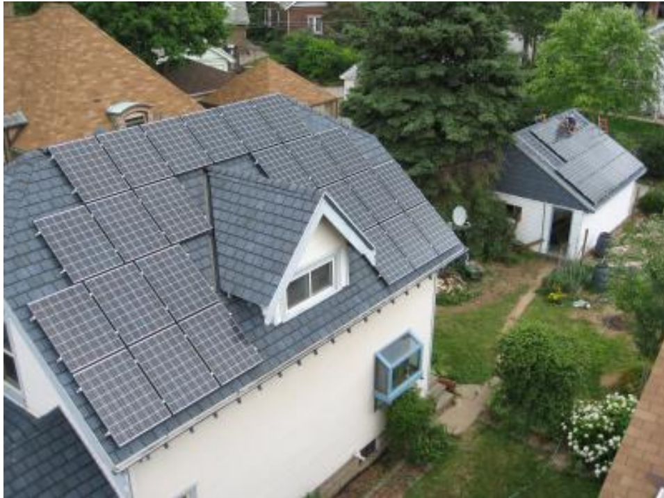
Solar panels on a Milwaukee home
