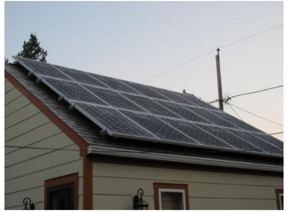
Example of rooftop solar
