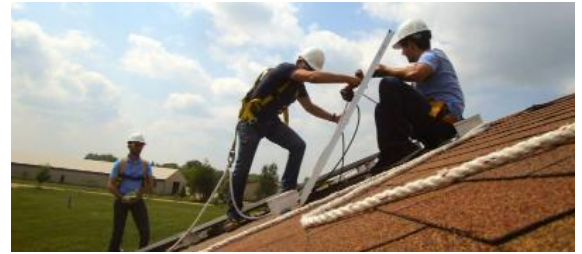
Midwest Renewable Energy Association solar installation
