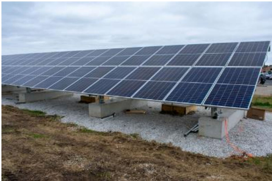
Closeup of Solar Now landfill array
